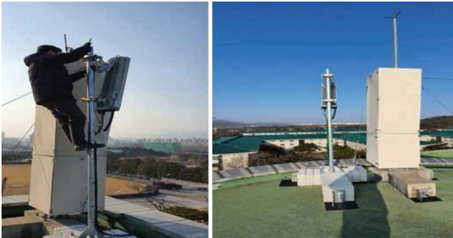
<Figure 3> 5G Network Base Station Installation (Shin et al. , 2020)
